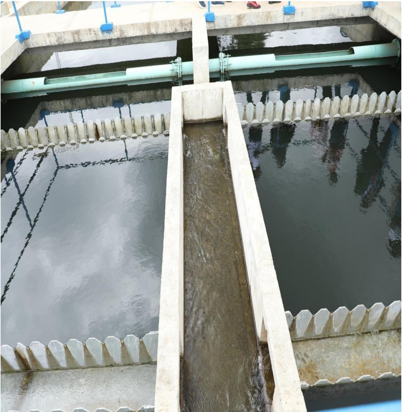
THE WATER TREATMENT PLANT
